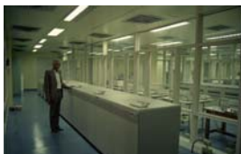
HP Servers (photograph dated 1990)
