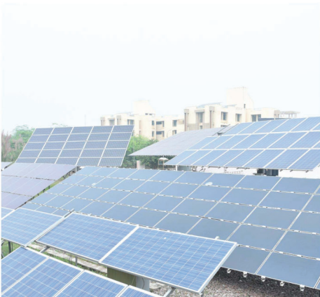
SOLAR PHOTOVOLTAIC POWER
