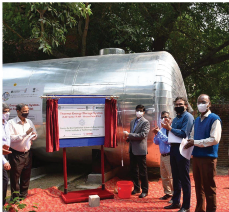
775 TR HR ENERGY STORAGE SYSTEM
