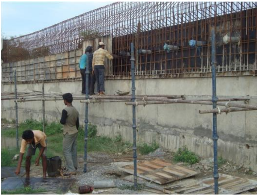
A view of wall formwork- the unsafe scaffolding
