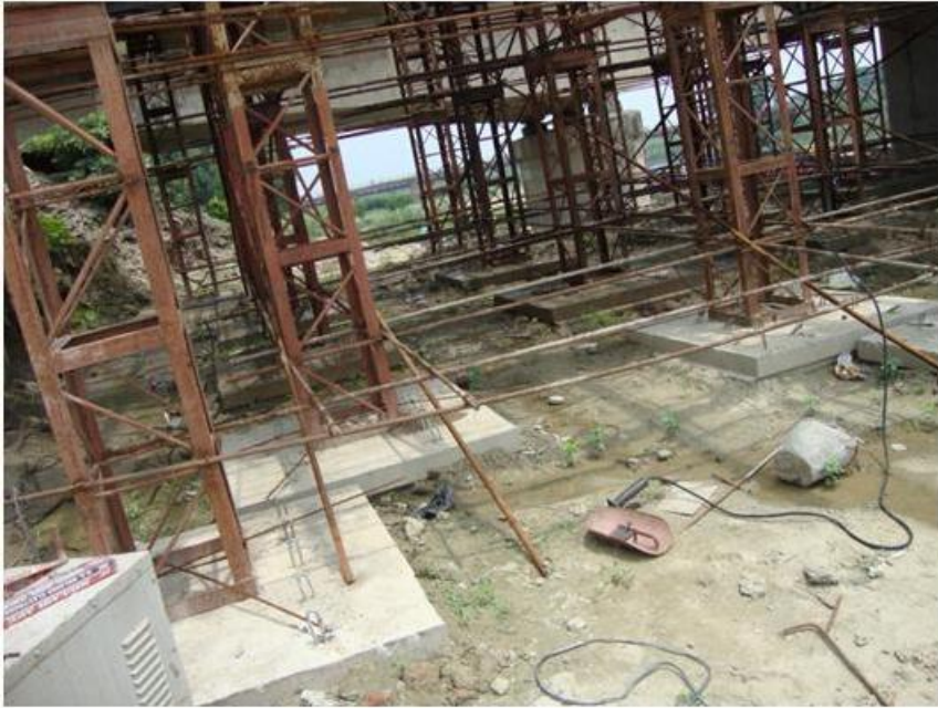
A view of bridge formwork- No trestle is anchored
