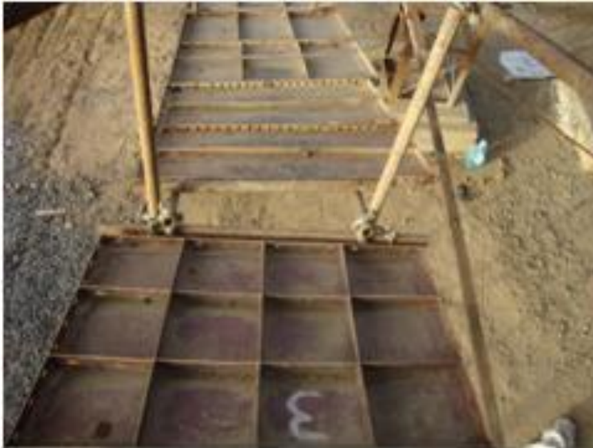
A view of access to workplace- misuse of shuttering plate
