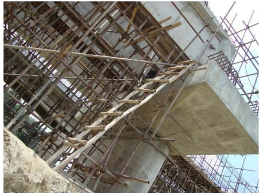
A view of bridge formwork- All safety norms violated
