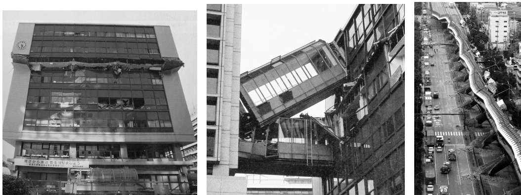
Photograph 1 Kobe City Office (from northwest, left), The Bridge of Kobe City Office (middle), Hanshin Highway (from north east, right)
