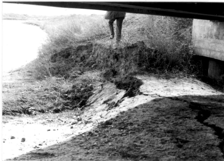
Photo 12 Embankment failure of a bridge over Karasu Çayı
