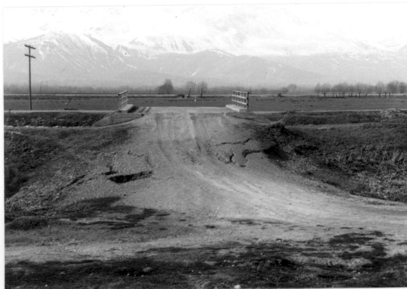
Photo 11 Embankment failure of a small bridge
