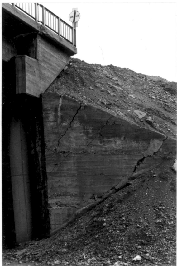
Photo 10 Fractured embankment walls of a cross-over bridge
