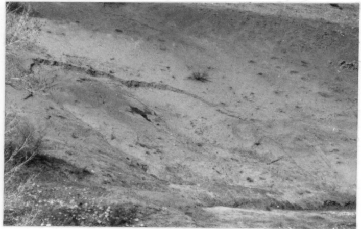
Photo 6 Soil slope failure near Tanyeri
