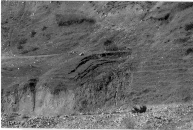
Photo 5 Soil slope failure near Tanyeri
