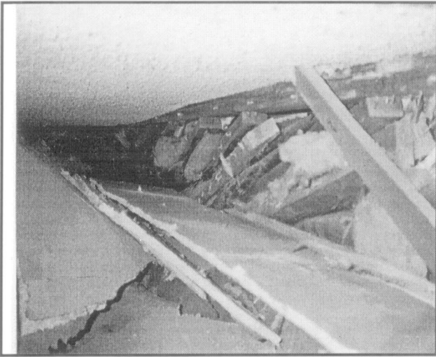
Figure 3. Within the 500 mm residual ground floor crawl space following collapse.
