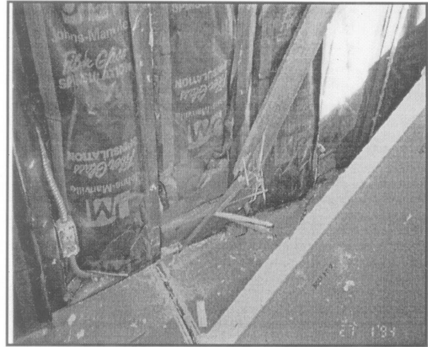
Figure 4 Compression brace failure and loss of sheet lining nearing collapse.
