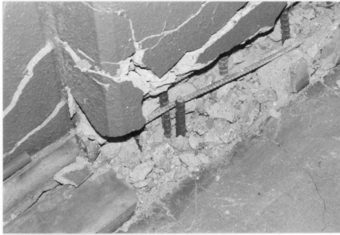
Photo. 2 The first story column destruction
