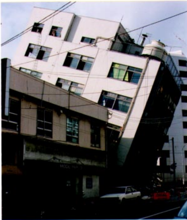
Fig.6. Class D building with grade 5 damage.
