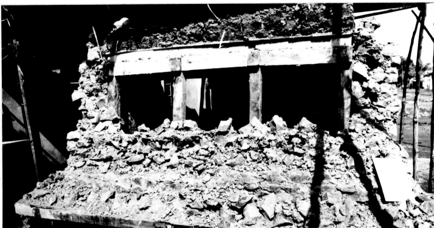
Fig. 2. Delaminated wall (Arya 1995)
