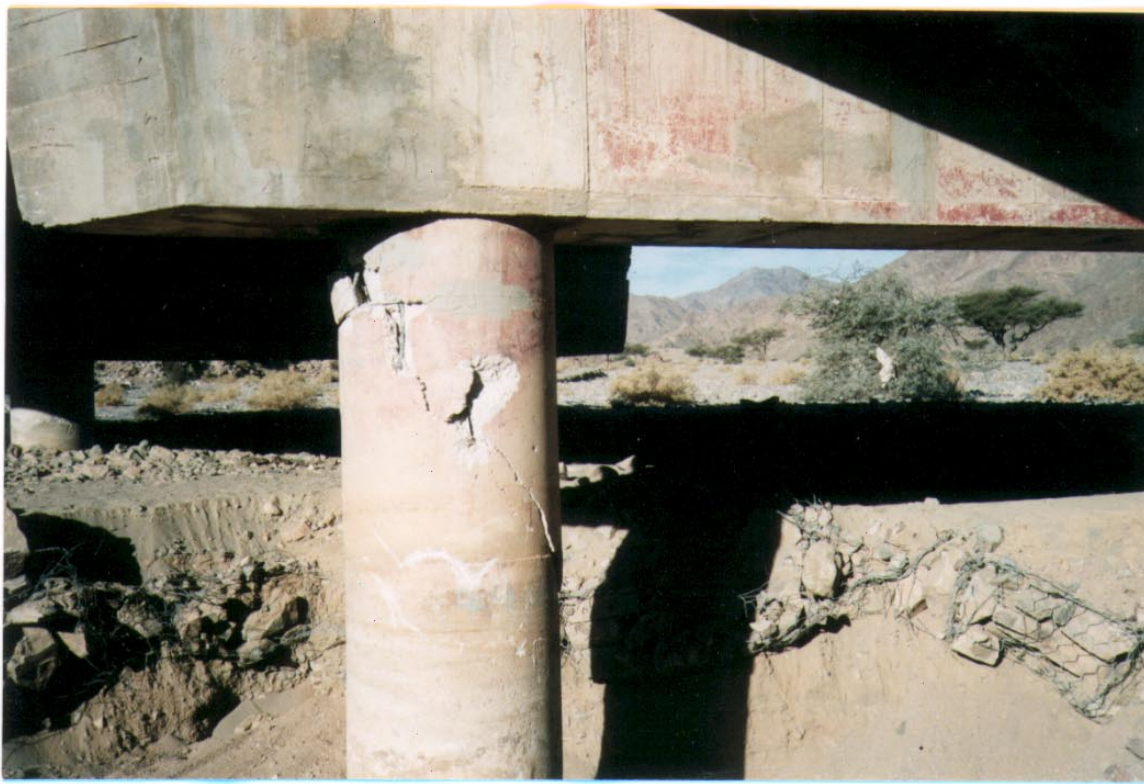
Fig. 8. Severe damage in columns of a main bridge
