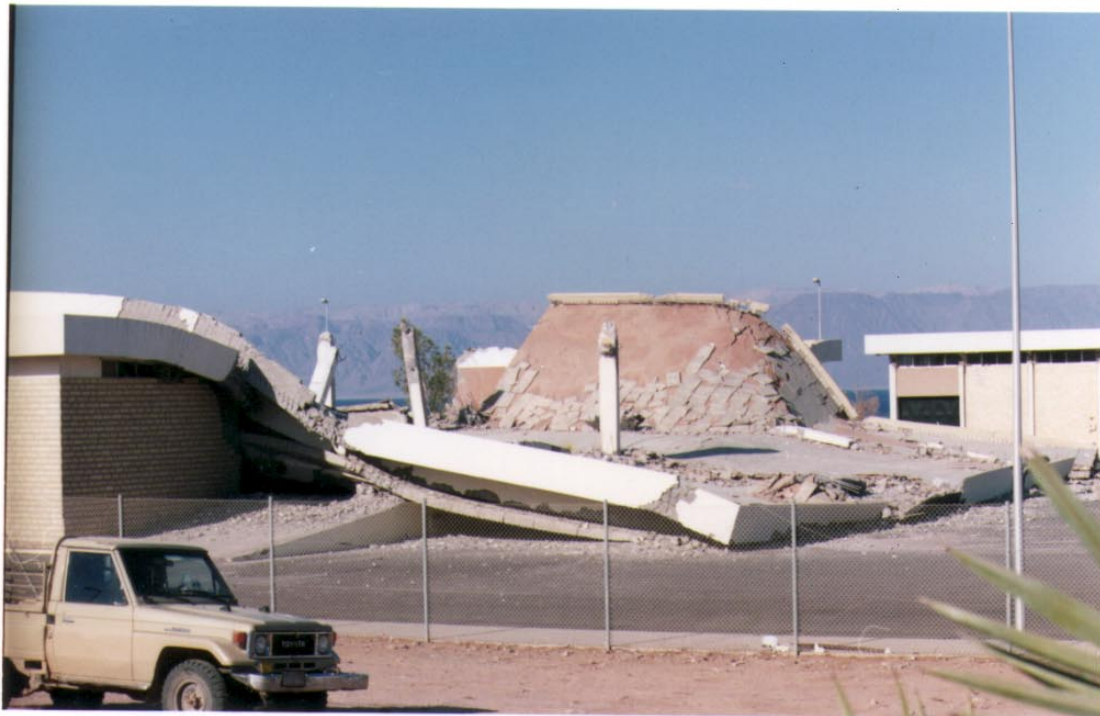
Fig. 7. Reinforced-concrete sheds completely collapsed in Ad Durrah customhouse
