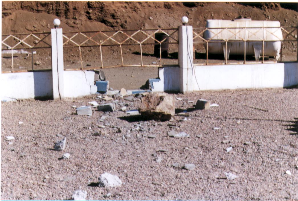
Fig. 3. Fence wall of a coast guard center damaged by fallen rocks
