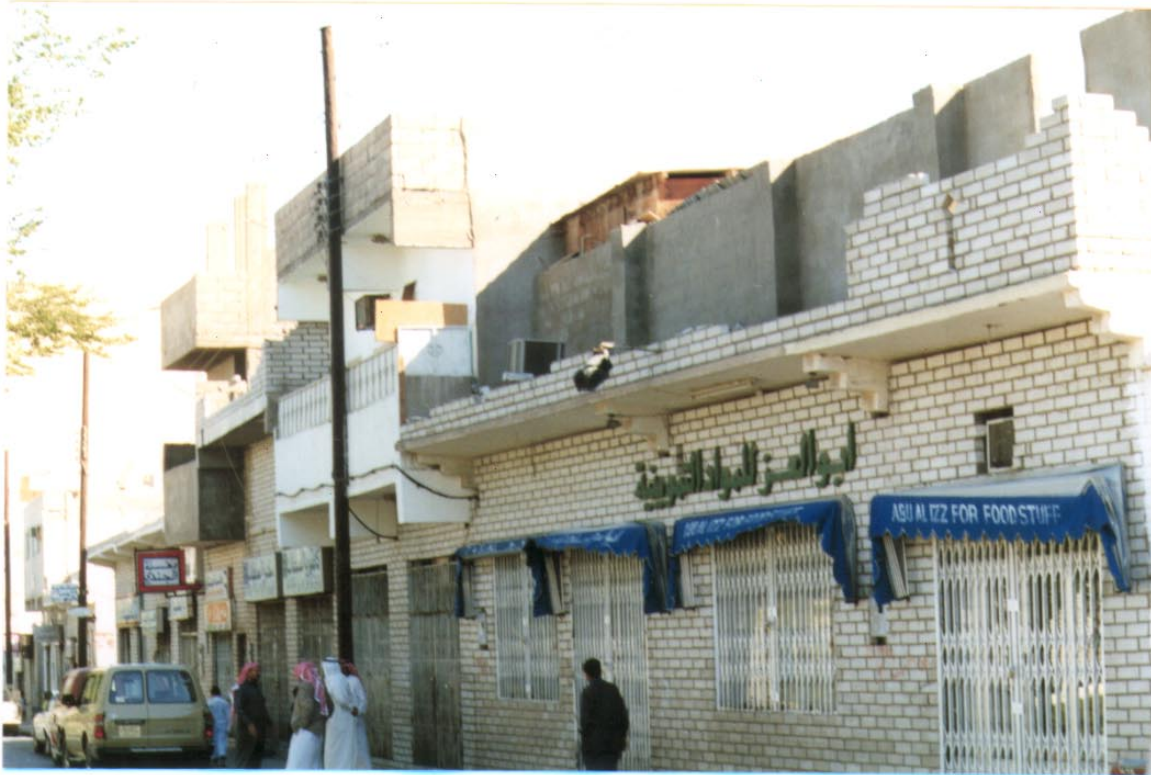
Fig. 5. Sand brick parapets fallen in downtown of Haql
