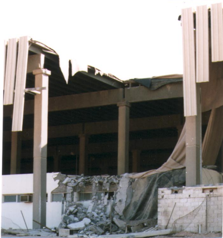
Fig. 6. Precast concrete shed partial collapsed in Ad Durrah customhouse
