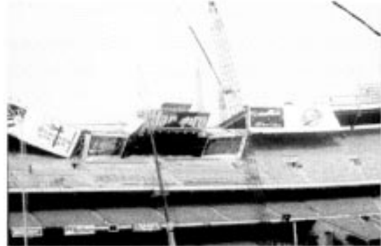
Fig. 6 Scoreboard collapse in stadium
