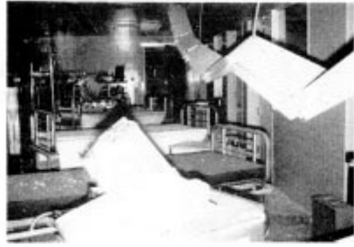
Fig. 3 Collapsed light fixtures (After Stratta, 1987)
