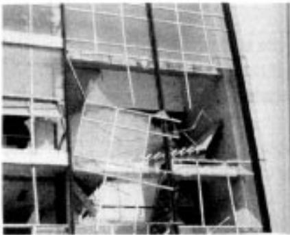
Fig. 4 Damage to cladding components (After Lagorio, 1990)
