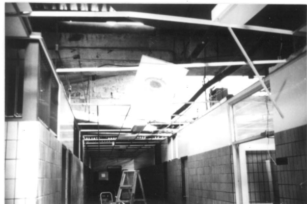
Fig.2 Hospital evacuated due to severe secondary damage after the Limon, Costa Rica, 1991 earthquake.
