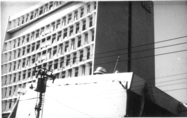
Fig.5 Benjamin Bloom Hospital, San Salvador. Collapse of two three-floor frame structures, while the eleven-floor tower that included structural walls remains standing.
