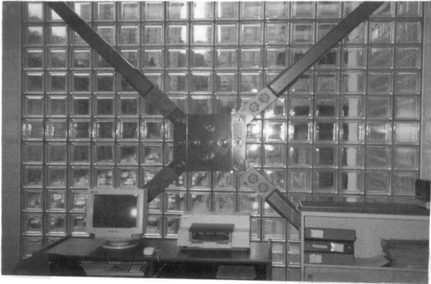
1 (b). Exposed Friction-Damper in Library Office
