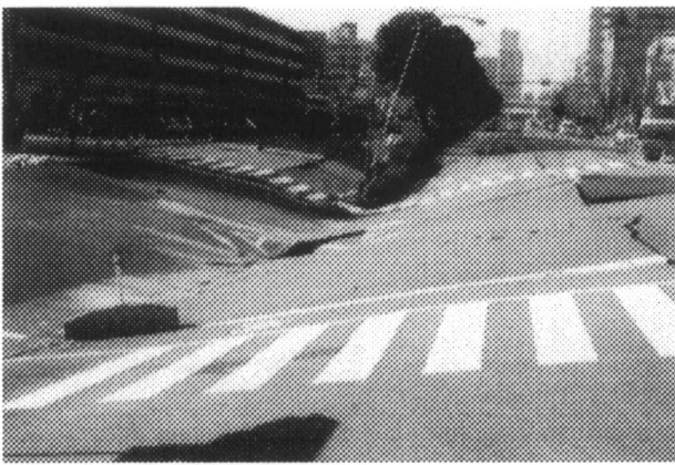
Photo.1 Subsidence of the pavement occurred over the subway station
