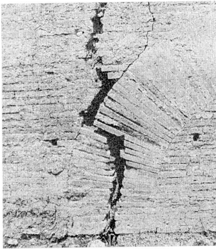
(a) vertical cracking of basilica wall at the Domus Flavia (c. 92 A.D.)
