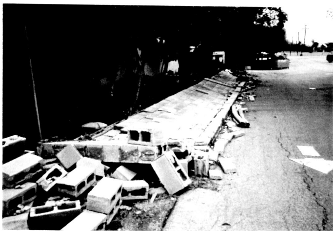
Fig. 2. Damaged wall and masonry units.
