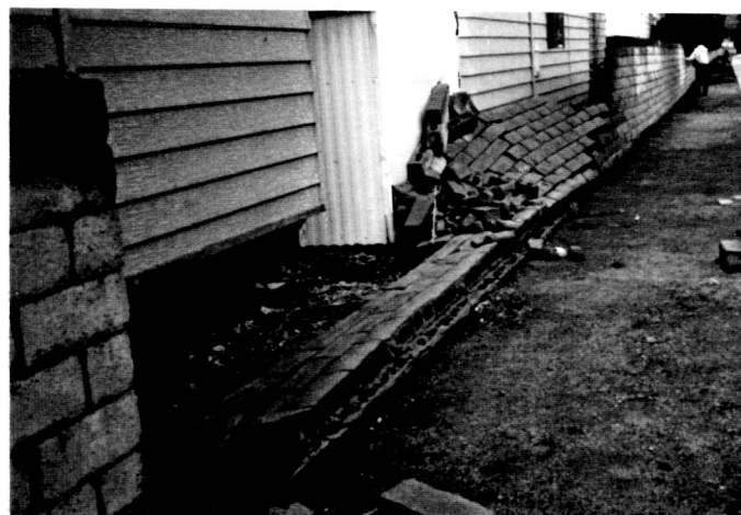
Fig. 3. Masonry wall without foundation.
