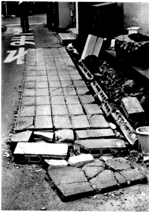
Fig. 9. Masonry wall without foundation.
