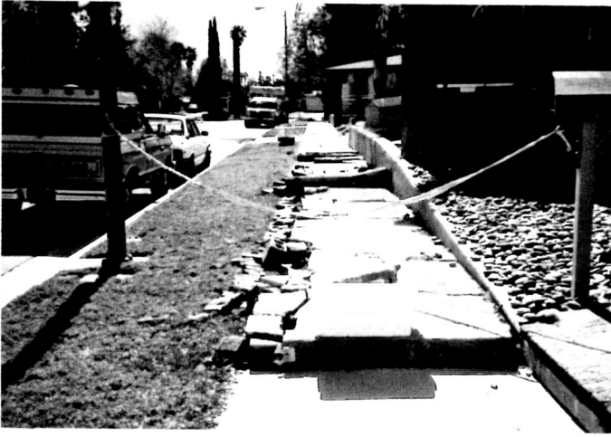
Fig. 4. Inadequate anchorage for vertical Re-bars.
