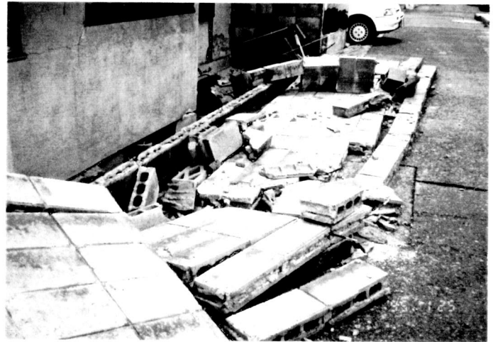
Fig. 12. Insufficient wall reinforcement.
