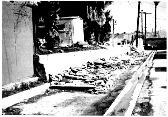
Fig. 5. Damage due to earth pressure.
