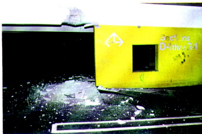
Fig. 6: Foundation failure limited effectiveness of shear wall
