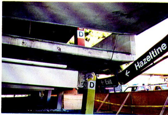
Fig. 8: Column damage related to proportioning deficiencies
