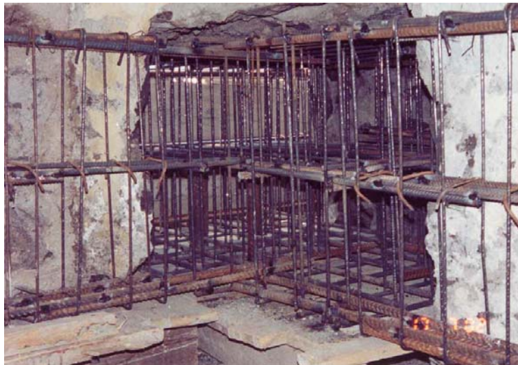
Figure 7. The view of the upper reinforcement frame installed in the opening together with the isolator upper socket after casting the concrete of the lower pedestal
