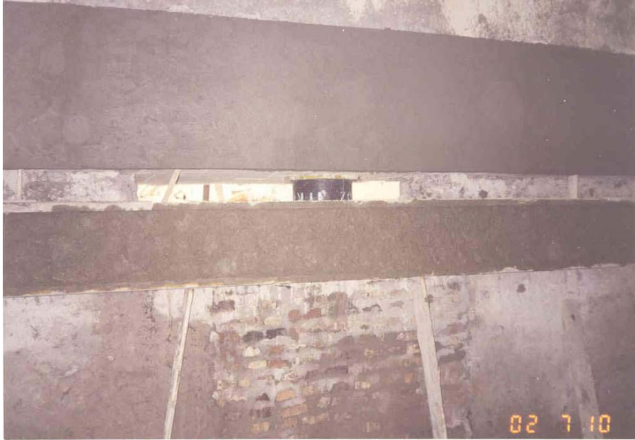
Figure 8. The view of a two-stage system of R/C continuous beams, which separate the building from its foundation and create the seismic isolation system
