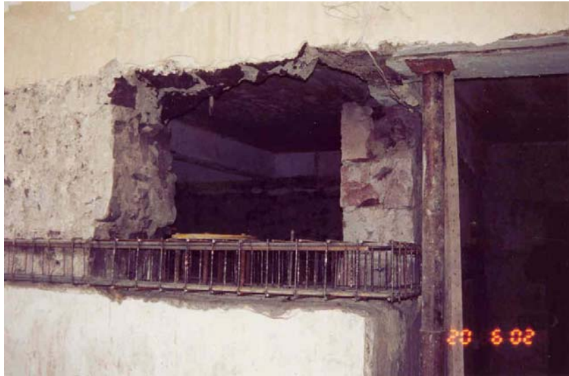
Figure 6. The view of the lower reinforcement frames installed in the opening together with the isolator socket
