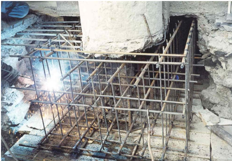
Figure 9. Existing column and the wall behind it are supported temporarily and the reinforcement frame of the upper pedestal is installed
