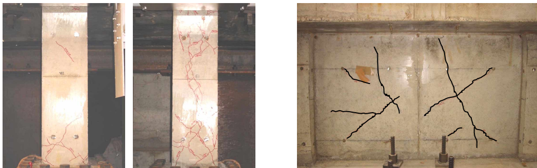
Figure 7 Crack pattern developed in columns and wall after JMA50
