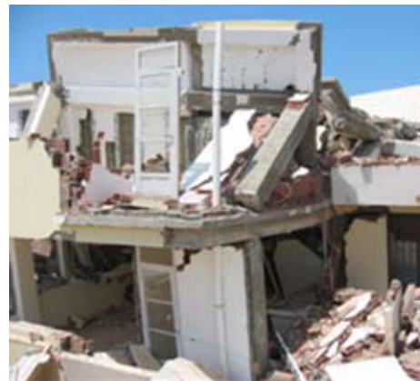
Photo 4.4: Poor concrete quality and execution
