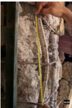
Photo 4.5: Non adequate detailing
