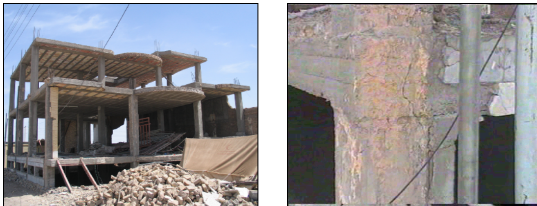
Figure 6 General view and cracking in beam-column connection zone of building RC2
