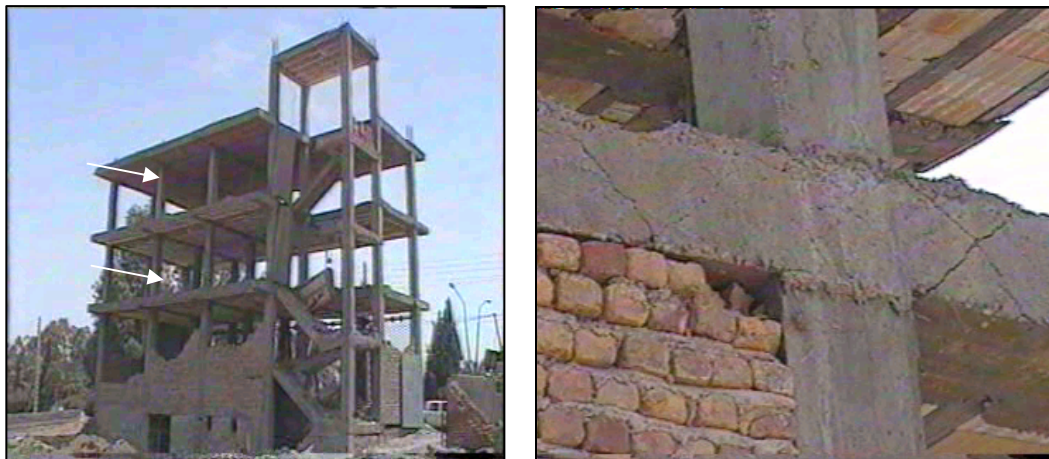
Figure 5 General view and diagonal cracks in beam elements of building RC1
