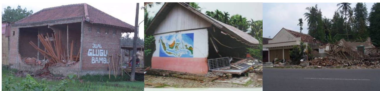
Figure 5. Damages in non-engineered buildings
