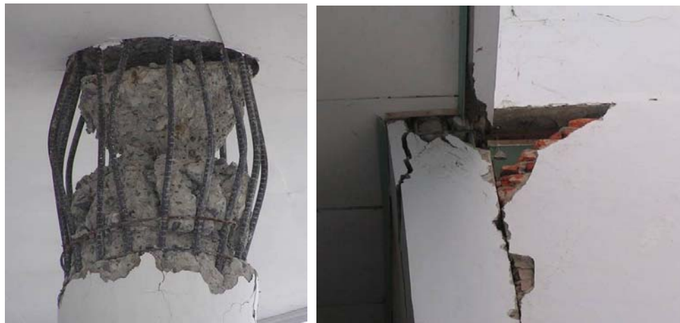
Figure 3. Failed elements and connections.
