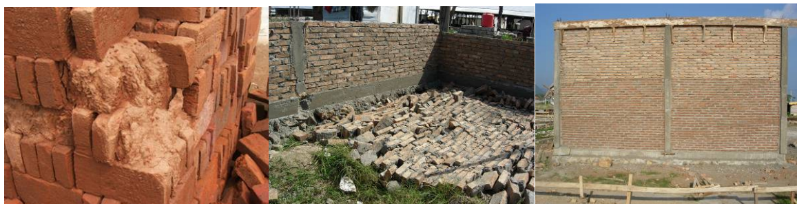
Figure 9. Poor material quality and workmanship, variation of brick quality found in Aceh reconstruction.
