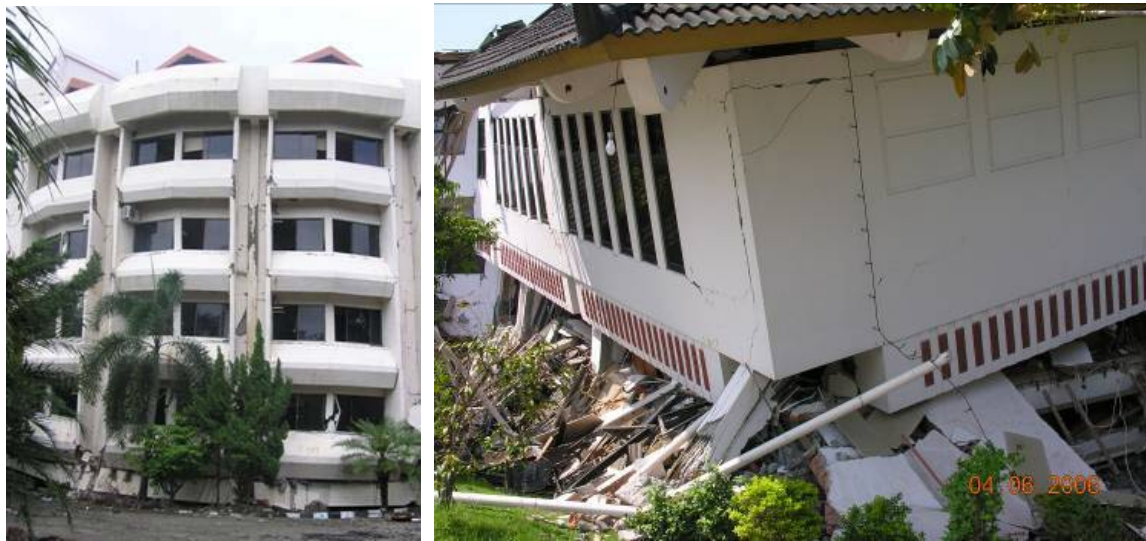
Figure 2. Soft story and weak story effects causing total collapse of structures
