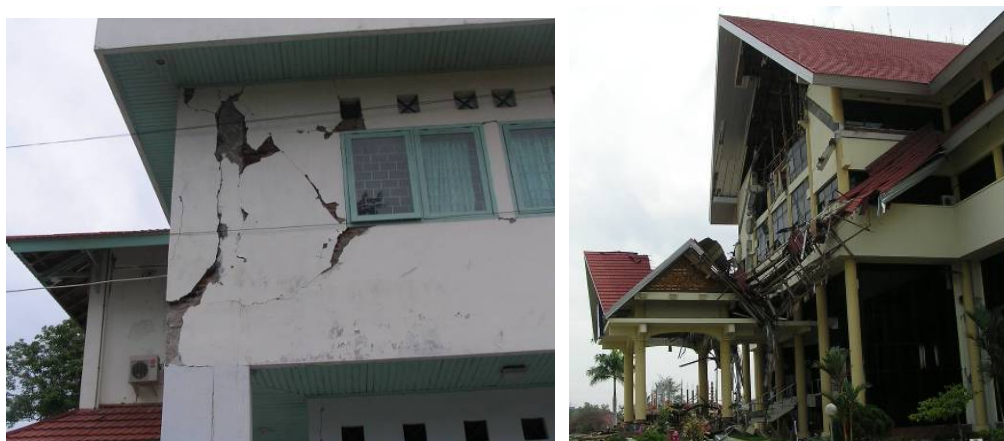
Figure 4. Failed elements and connections.
