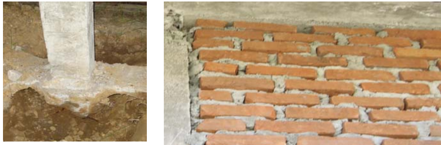
Figure 5. Missing foundation under column and brick detail
