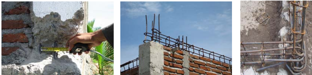
Figure 4. Incorrect stirrup dimension and joint details
