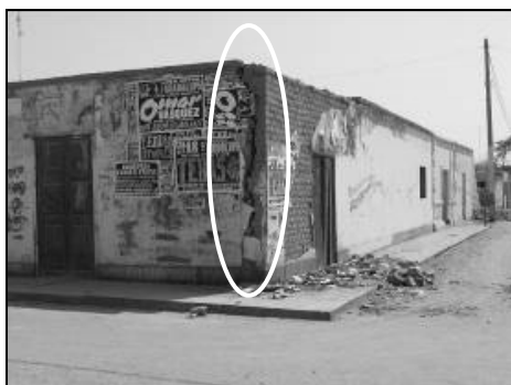
Figure 4 Vertical cracks in the wall's corner.
