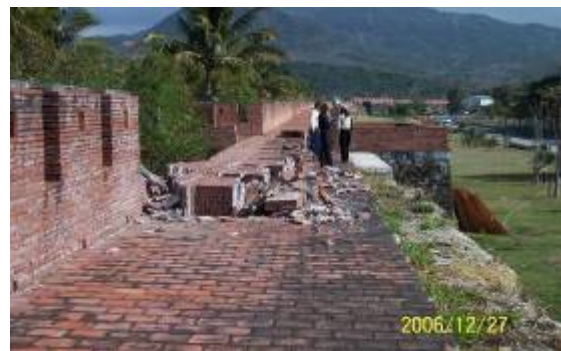
Fig.6 Hengchun ancient city wall collapsed
