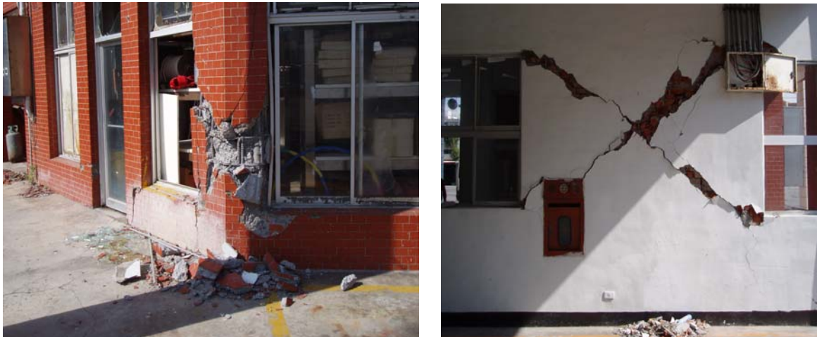
Fig.2 Structural damages on Taitung county fire bureau building
