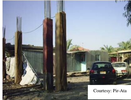
Figure 7 Two columns positioned very close together indicate inappropriate structural design
