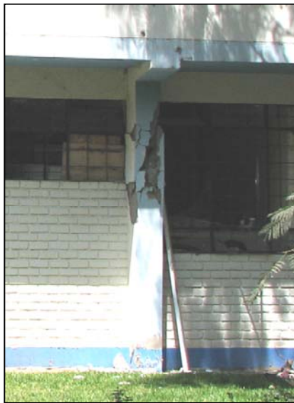
(a) Shear failure, CW18
