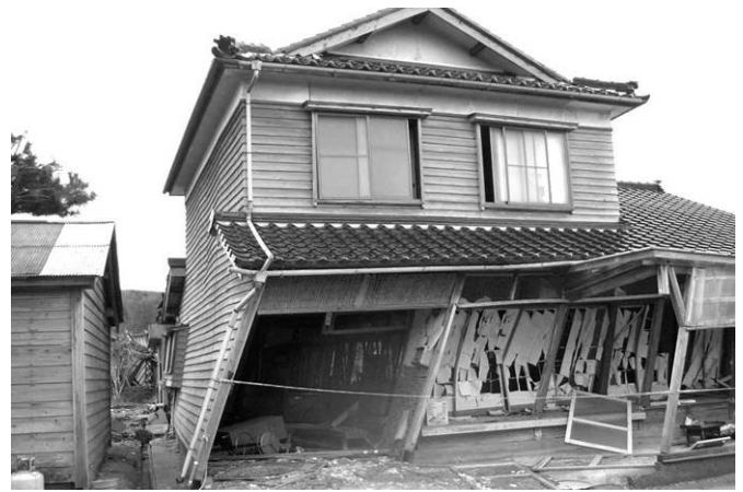
Photo 1. Typical damage to wooden house
