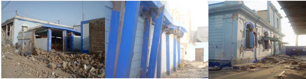
Figure 3. Structures of adobe and reinforced concrete with very severe damage and collapse.
