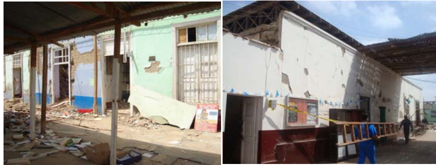
Figure 4. Severe Damage in old buildings of the hospital
