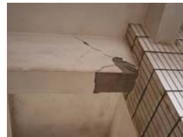
Fig. 15 Damage of beam end
