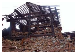
Fig. 7 Walls collapsed & wooden frames standing
