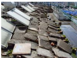
Fig. 14 Damage of thermal insulating layer
