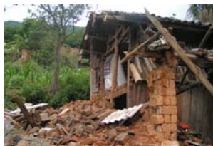
Fig. 6 Wooden roof truss collapsed
