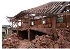
Fig. 8 Integral collapse of wooden structure
