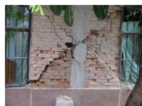
Fig. 11 X cracks on wall between windows
