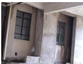
Fig. 16 Shear damage of ground floor column
