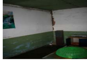
Fig. 13 Junction crack of walls
