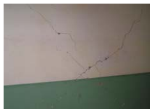
Fig.10 Oblique cracks on load-bearing wall
