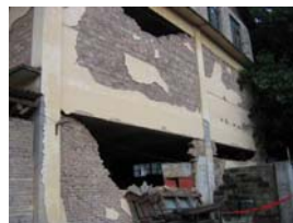
Fig. 17 Damage of filler wall
