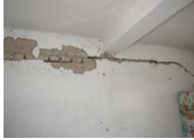
Fig. 12 Horizontal cracks on load-bearing wall
