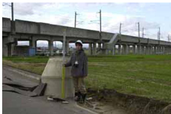
Photo 1 Uplift of manhole and settlement of pavement above backfill soil for pipe
