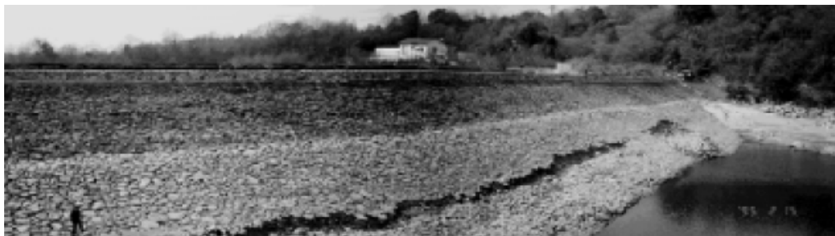
Figure 1 The sliding failure zone in Kitayama dam caused by Kobe 1995 earthquake
