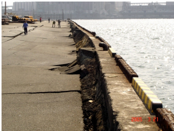
Figure 1 Large seaward displacement of quay
