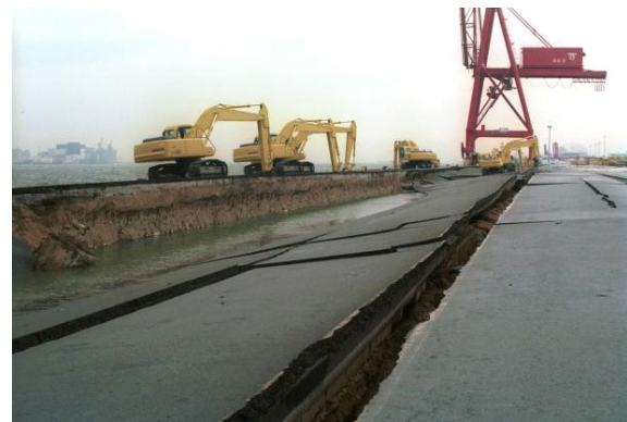
Figure 2 Large settlement of backyard ground
