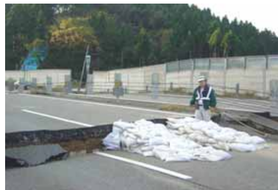
Photo 3 Differential settlement between embankment and culvert at C-Box Kawaguchi 11
