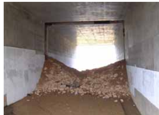
Photo 5 Separation of joint at C-Box Ojiya 2
