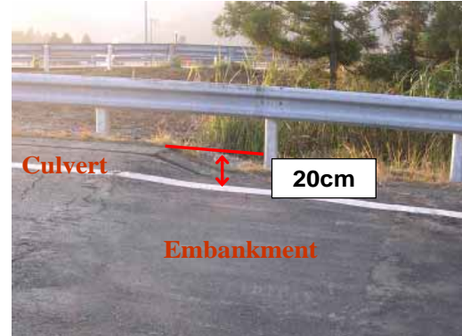
Photo 4 Differential settlement at C-Box Kawaguchi 22
