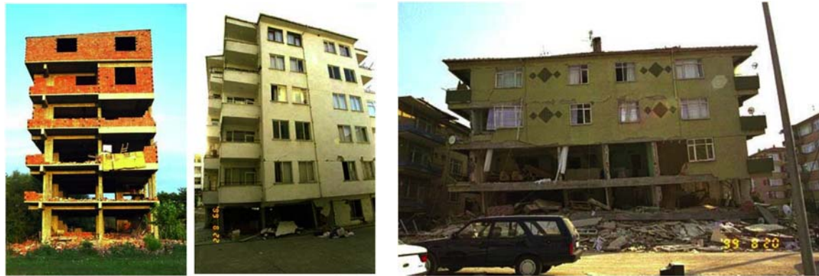
(a) Damage to masonry infill walls (b) Failure of building frame with masonry infill Figure 1 Damage of moment resisting frame building
