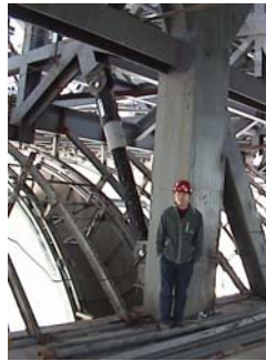
Fig.7 Installed 1500kN Damper
