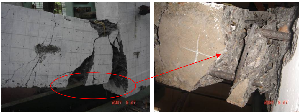
(b) Bottom steel rupture of B4 near the column
