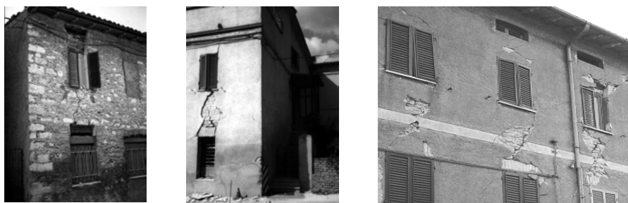
Figure 1. Some examples of earthquake damage in existing un-reinforced masonry buildings
