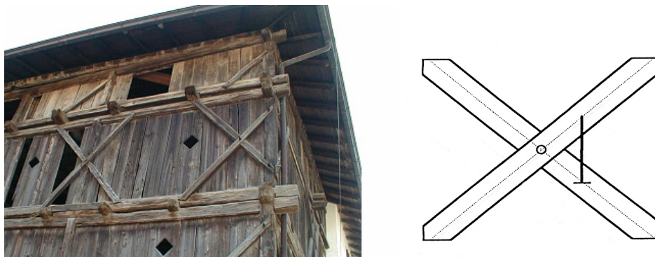
Figure 3. Half-depth cross joint in bracings of a timber structure (left); scheme of the jointed elements in a specimen, the vertical bar indicates the position of relative displacement measures (right)
