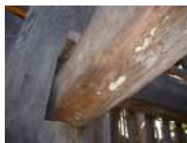
Photo. 1 Deteriorated beam-column joint
