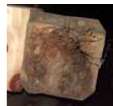
Photo. 2 Column with internal loss
