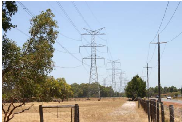
Figure 1. Transmission towers located in the northeast of PMA
