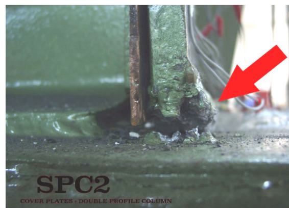
Figure 7. Specimen 2- Complete cracking of weld root adjacent the Copper Back weld plate
