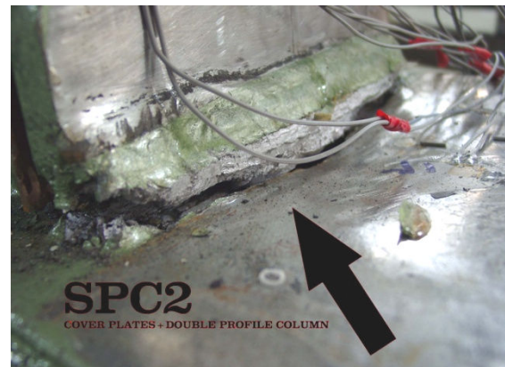
Figure9. Specimen 2- Through the thickness crack propagation in the end plate
