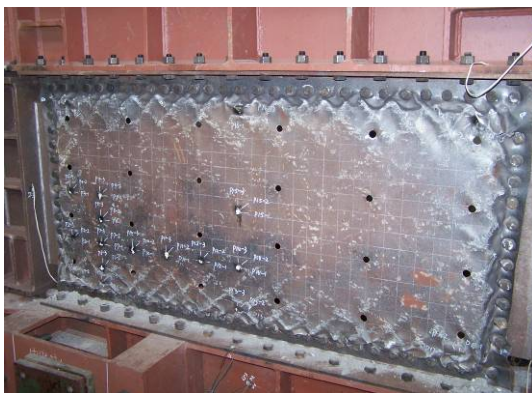
Figure 4. Residual deformation of the steel plate in the CSPW specimen (Gao 2007)
