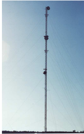
Figure 1. Example of a 111.2 m guyed tower located in St. Hyacinthe, Québec, Canada
