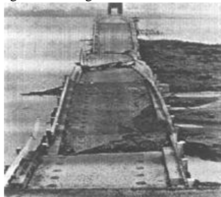
Fig.6 pile body sinking, Copper highway bridge, Alaska earthquake, 1964
