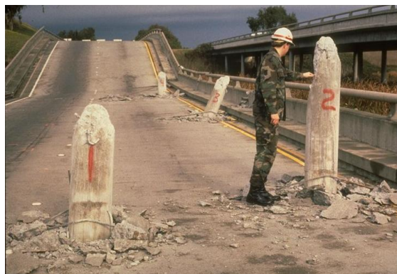
Fig.7 piers penetrate bridge deck, Struve Slough bridge, Loma Prieta earthquake, 1989
