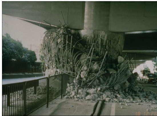
Fig.1 Crushing failure , Hyogoken-Nanbu earthquake
