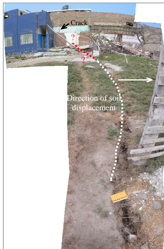
Figure 2. Soil displacement crack next to old building. The crack probably continues in front of and/or beneath the building and then up through the confined masonry wall as marked by the black arrow. (The curvature of the building top is due image distortion, it should be a straight line.) The sewage system in Pisco, whose conditions were already poor before the earthquake, was drastically affected
