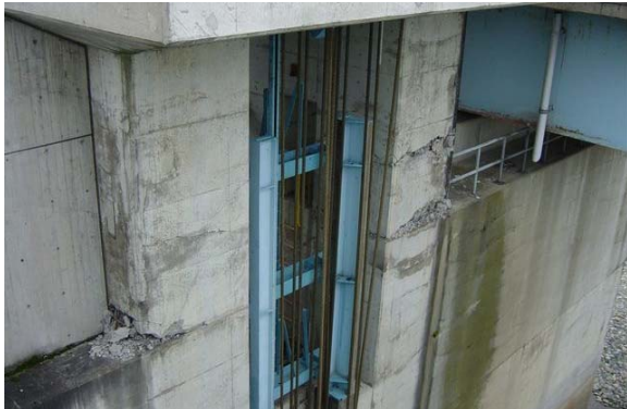
Picture 1 Damaged Gate Column of Myoken weir by 2004 Mid-Niigata Earthquake
