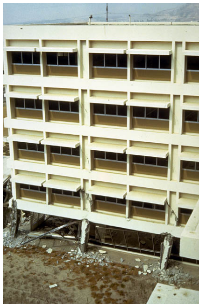
Figure 1 Damage due to a soft story at the ground floor in a multi story building during San Fernando earthquake in California, 1971
