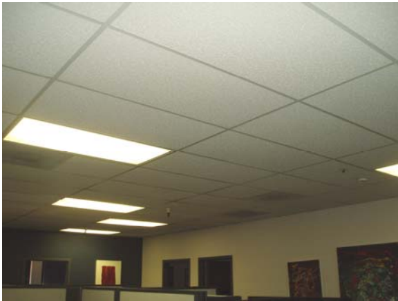
Figure 1. Suspended ceiling in an office building
