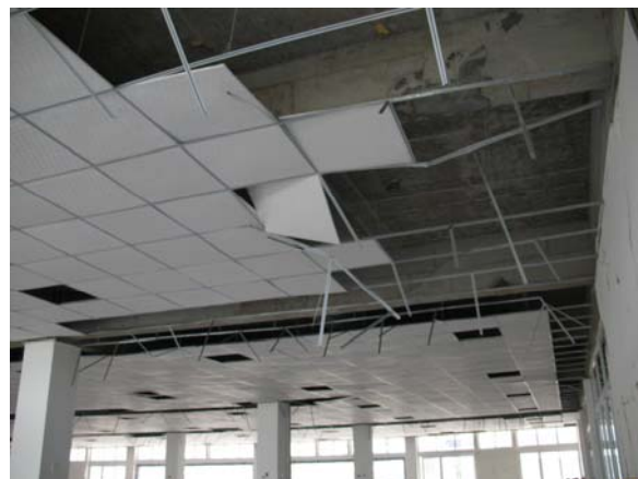
Figure 4. Ceiling damage Sichuan (China) 2007
