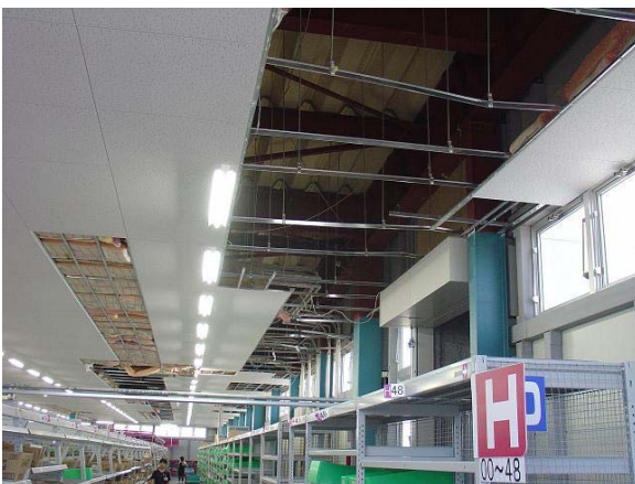
Figure 3. Ceiling damage Niigata (Japan) 2007
