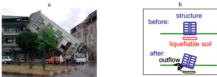
Figure 1: (a) Tilted and settled building in Adapazari (Peer 2000), (b) sketch of liquefaction underneath a building (Buchheister 2007)
